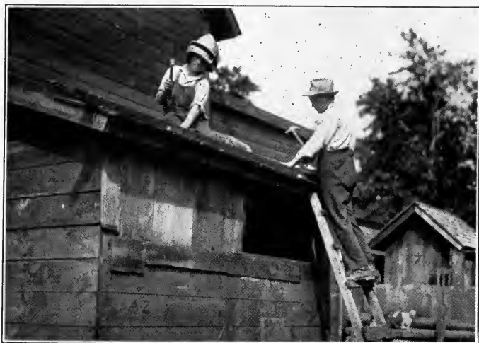
Shingling a roof. Ordinary practical work which is accompanied by a valuable trying-out process
